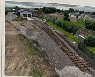
Tracklaying at the A1 Steam Locomotive Trust's new base at Darlington Locomotive Works continues, with the new headshunt taking shape but one of the areas still in need of ballasting. A1SLT
